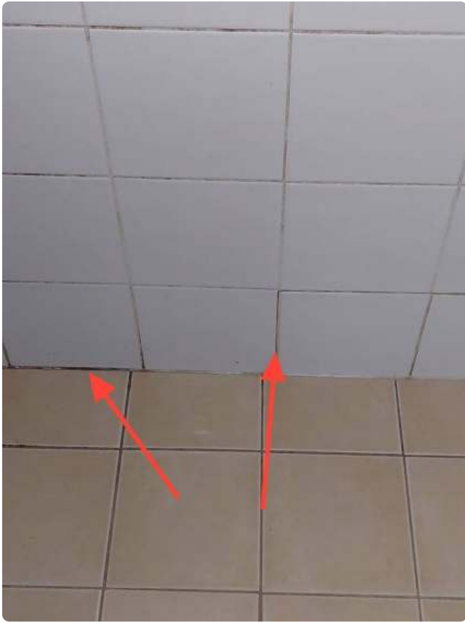
Grout missing in shower
