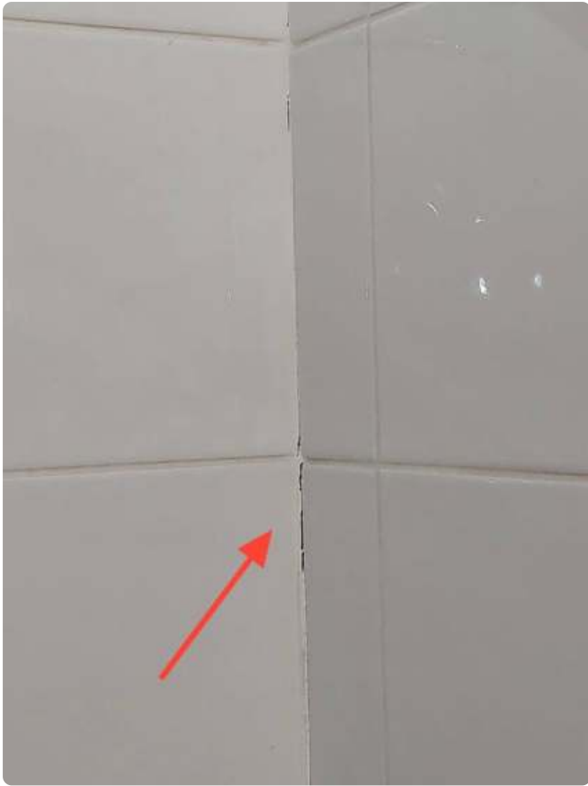
grout missing on shower wall
