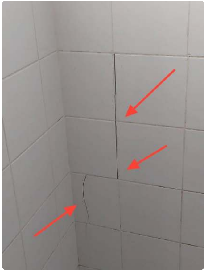
Tiles cracked in shower
